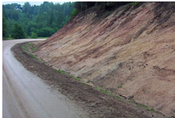
Figure 1: A steeply sloping side cut along the curved section of a highway (Photograph courtesy of ROADEX Network, Finland).
