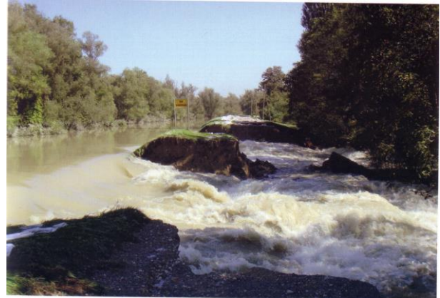
Figure 3: Breakage of the Sava embankment at Sop Bukevski on 19 September 2010.
